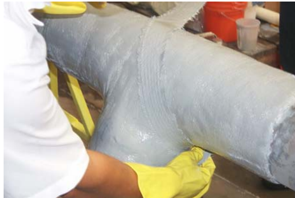
Figure 6 – Repair of pipe tee fitting using Armor Plate® Pipe Wrap 6-in standard wall tee with 50% corrosion Unrepaired burst pressure of 6,546 psi • Repaired burst pressure of 7,500 psi
