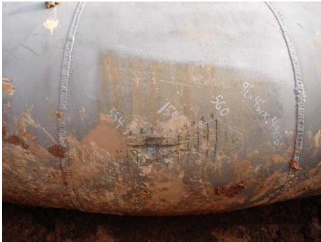
Figure 5 - Photograph showing corroded elbow
